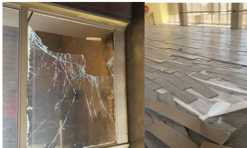
Window broken and the dance floor is flooded.
