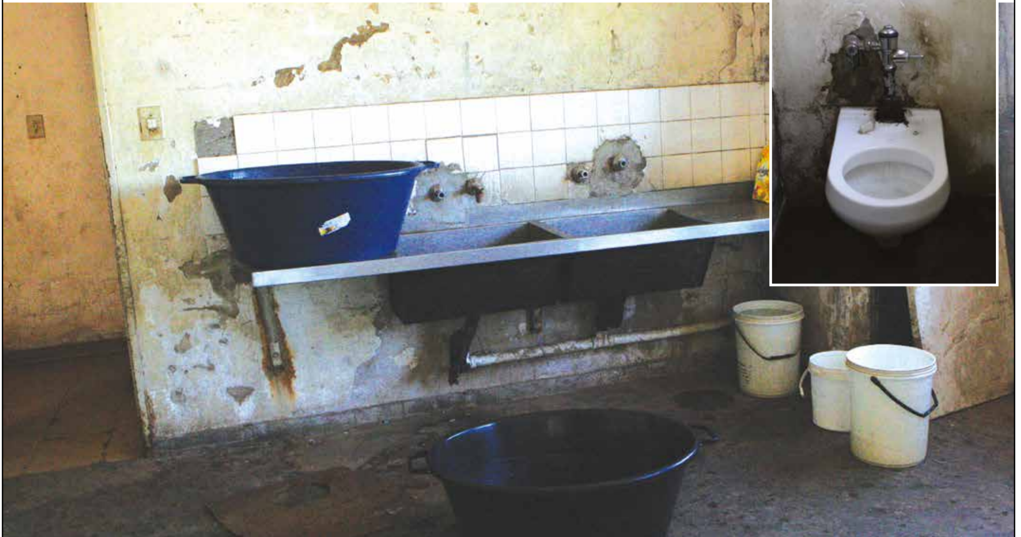
DEPRESSING: The deplorable state of the SAPS barracks in Soweto.
