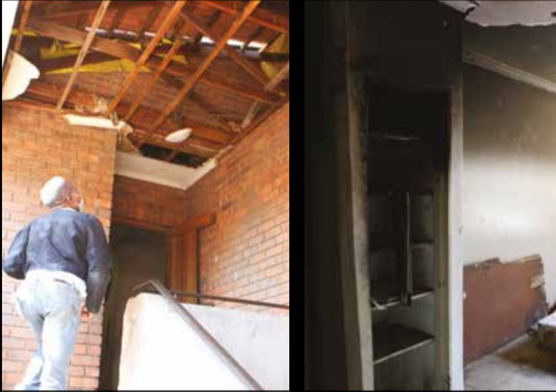
WeeklySAMirror senior journalist Thuli Zungu inspects the damage to the roof at a police apartment block.
